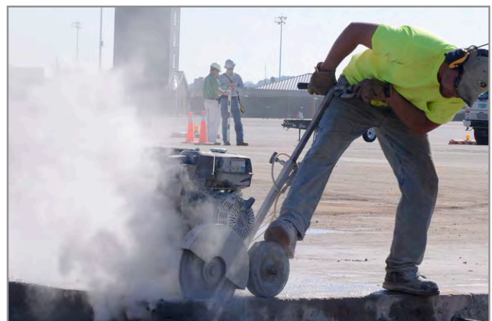
Contractors perform repairs to the Dobbins flightline taxiway A March 10. (U.S. Air Force photo/Don Peek)
